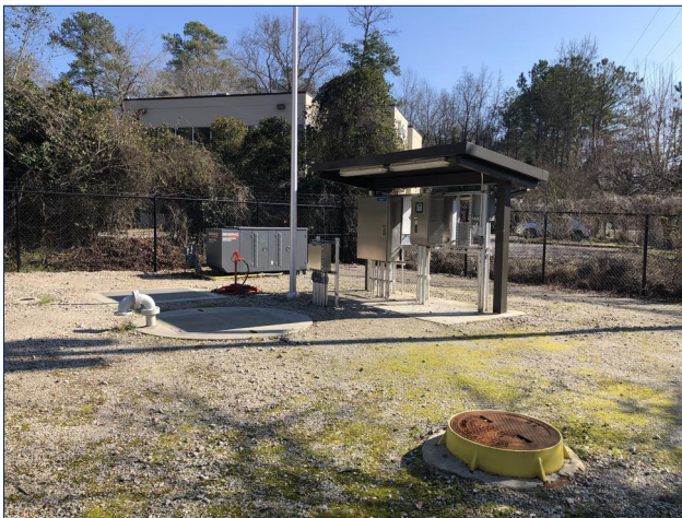
Figure 2-1 Existing CLPS to be Relocated
